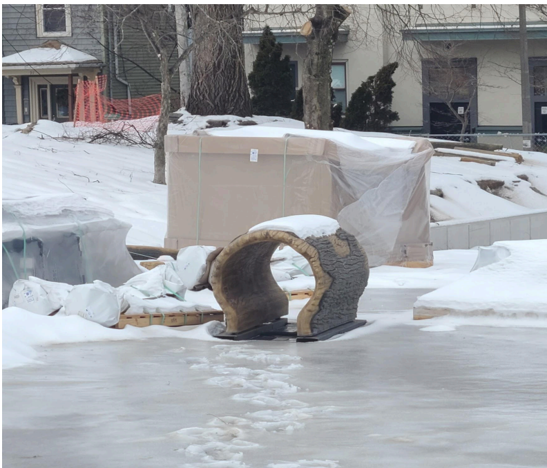
Play equipment on pallets and in boxes/packaging is now waiting on site for the ground to thaw enough so we can install footings (concrete bases) and install the equipment in the play area.
