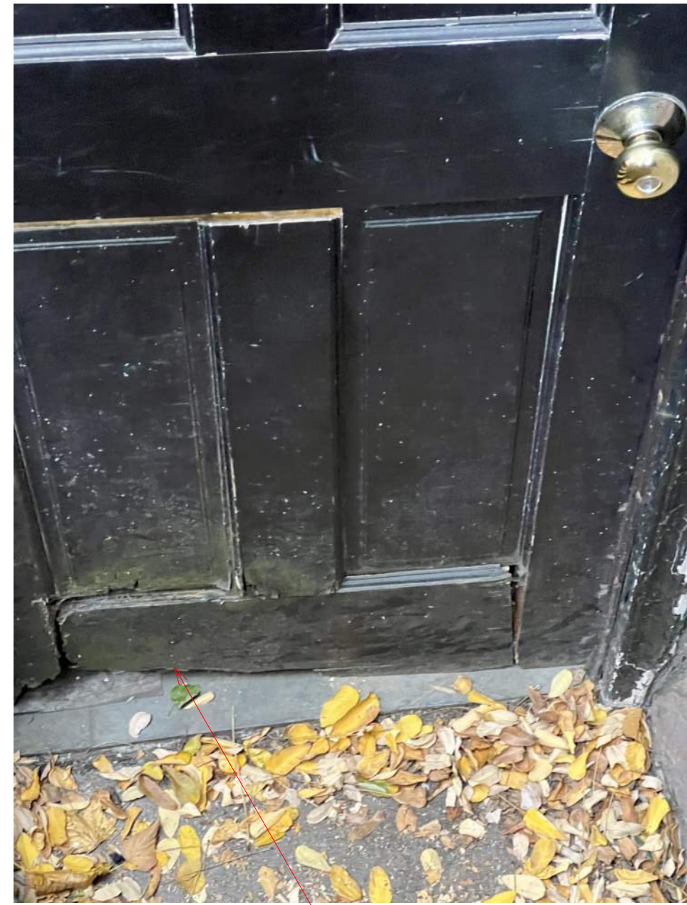
EXAMPLE OF WATER DAMAGED SIDE DOOR
