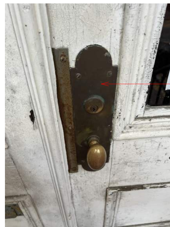
EXISTING BRASS FRONT DOOR KNOB, TO BE BUFFED AND POLISHED (OR REPLACED?)
