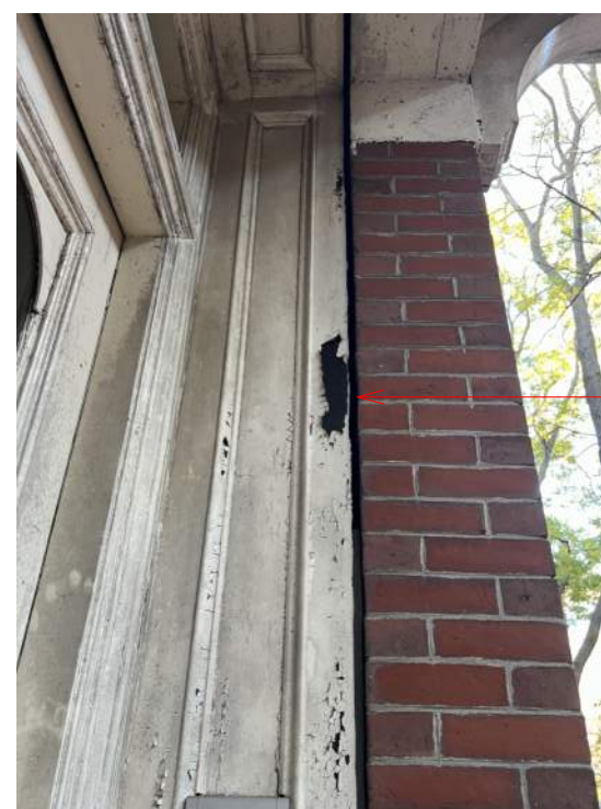
EXAMPLE OF PEELING/CHIPPING PAINT
