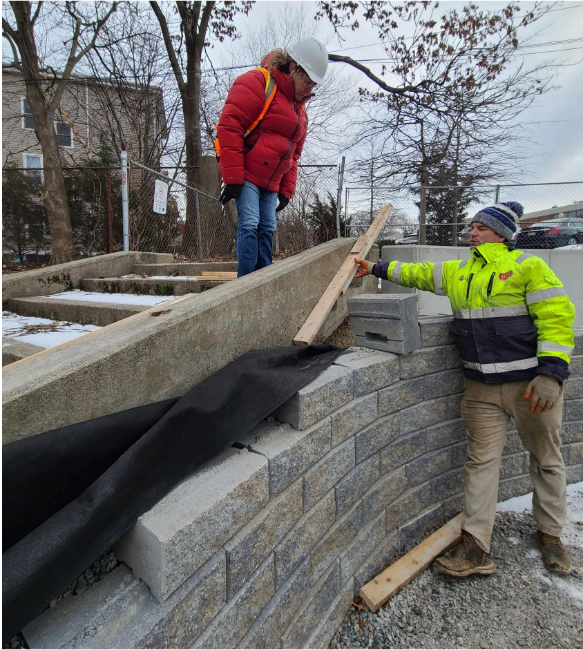
One of the unit block retaining walls, by the entrance near the Health Center. We are keeping these steps in place, so we need to determine how the new wall and existing steps work together.
