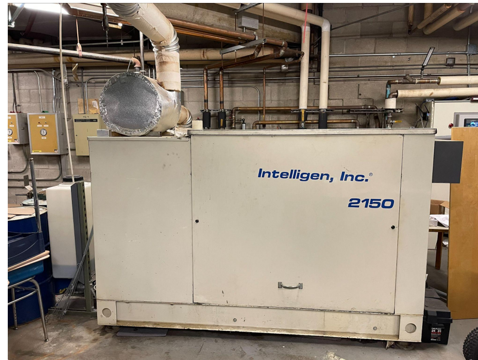
Ohrenberger School 250 kW Unit: Controls upgraded in Summer 2024 to allow for participation in demand response program and improved data tracking
