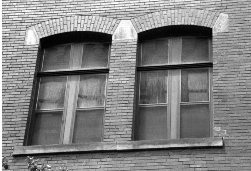
Fig. 21. Stilted arches, formed of a segmental arch with contrasting stils at the springing line. Photograph of 34-46 Farnsworth Street.
