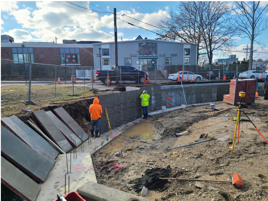
Play equipment will be installed at this new lower elevation, ensuring that we can make the park and playground accessible. A small bridge will connect the play equipment to the top of this wall. Gently-sloped pathways will allow park users to enter, along either side.
