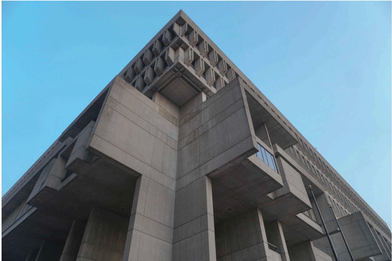
Figure 9. View under eaves at southeast corner, June 2023. Photo credit: Building Conservation Associates.
