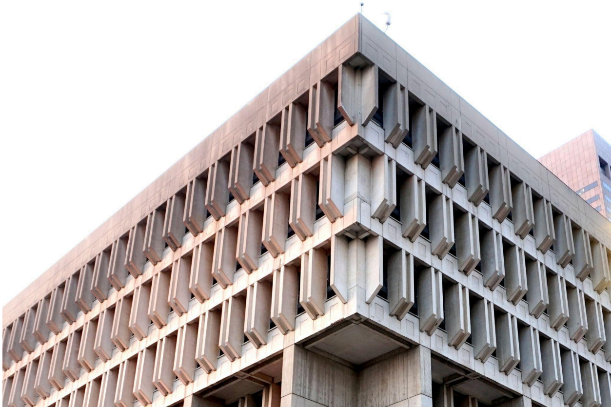
Figure 10. Crown detail (northwest corner) showing alternating windows and paired fins at upper (administrative departments) levels, June 2023. Photo credit: Building Conservation Associates.
