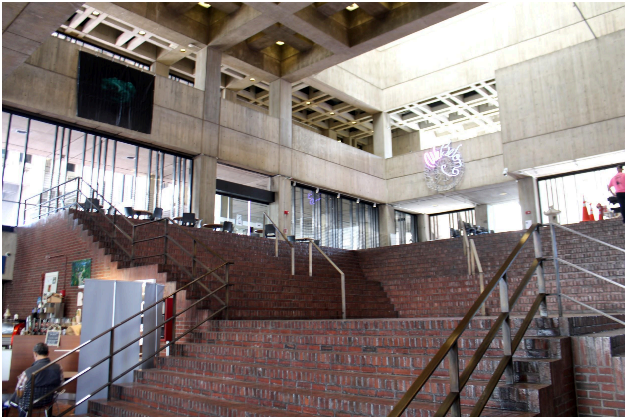
Figure 14. Main lobby, looking northeast from the third-floor entrance up the brick staircase towards the fourth-floor access to courtyard, June 2023. Photo credit: Building Conservation Associates.
