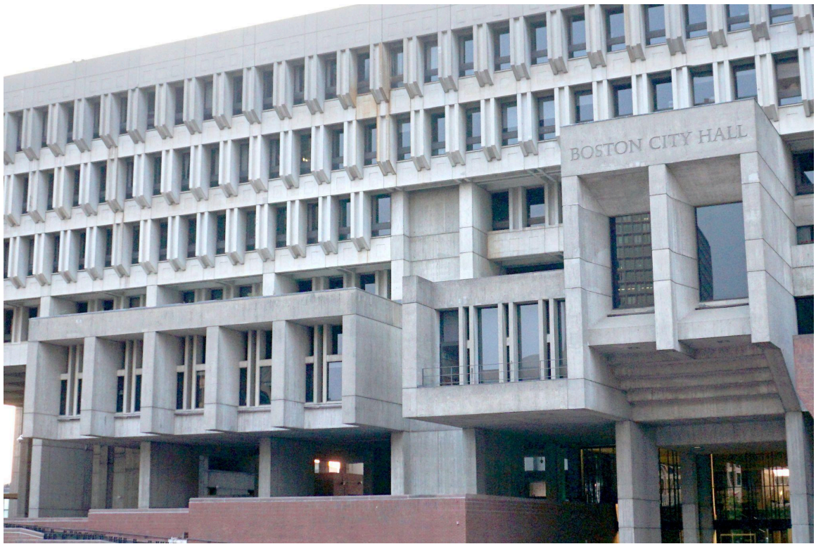
Figure 11. Cast-in-place concrete hoods for City Council offices (left) and City Council Chamber (right), June 2023). Photo credit: Building Conservation Associates.
