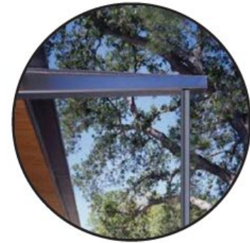
Roof scupper system painted steel
