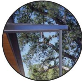
Roof scupper system painted steel
