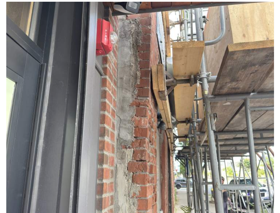
MASONRY WALL LEANING FORWARDS
