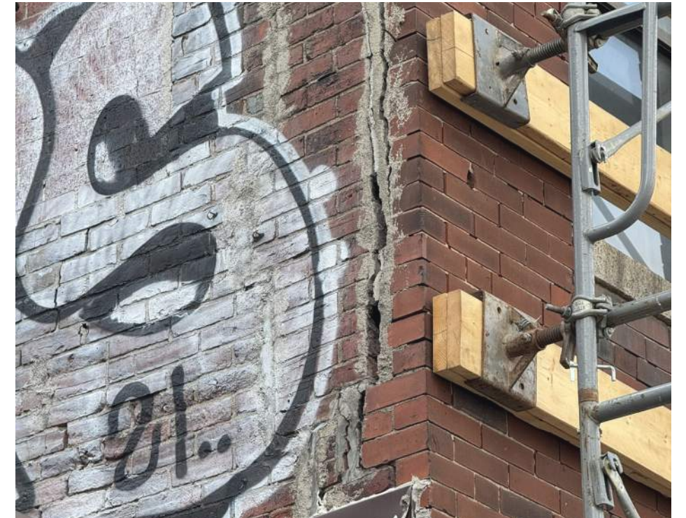
SEPARATION OF MASONRY WALLS
