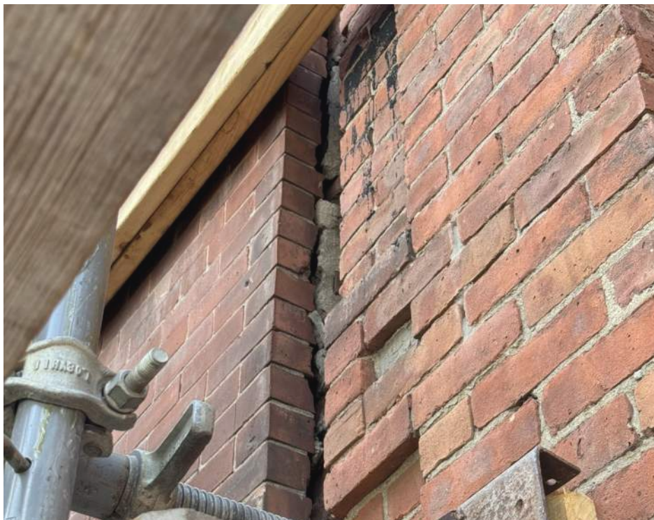
SEPARATION OF MASONRY WALLS
