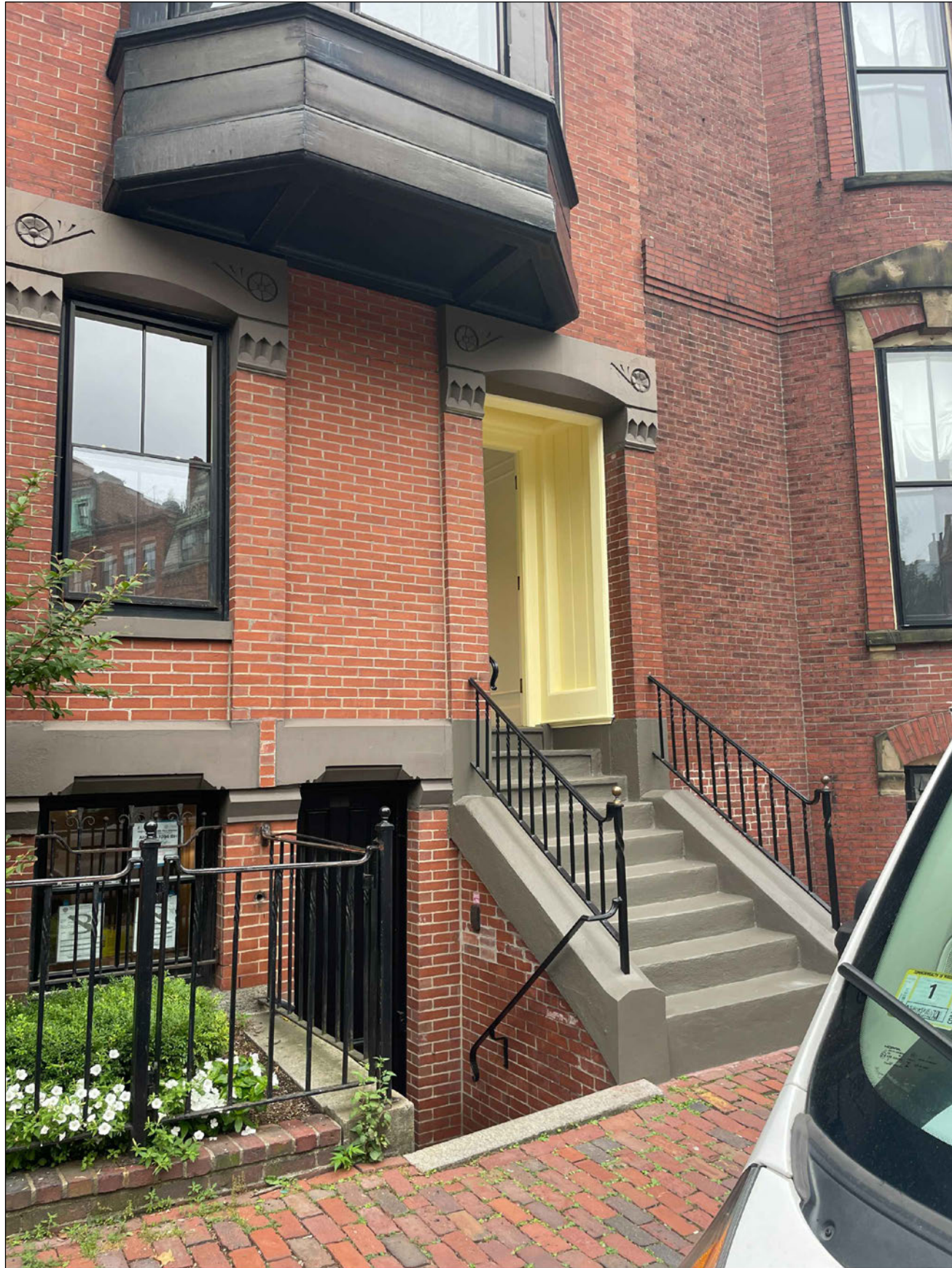
1 FRONT ENTRY (VISIBLE FROM MT VERNON ST) WITH PROPOSED EMERGENCY ELECTRICAL SHUTOFF
