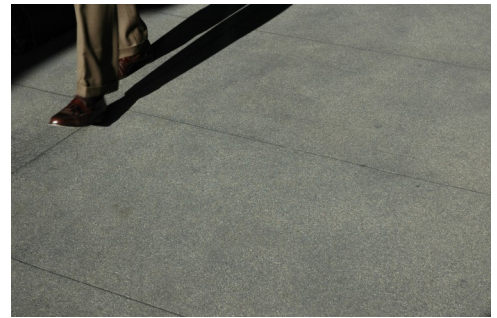
Example of a sidewalk with darker gray color, smooth finish and saw-cut joints.
