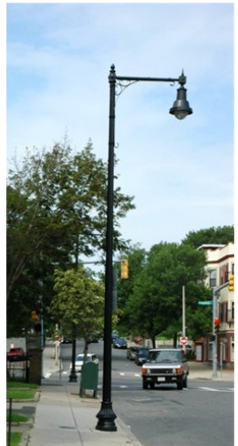
Example of pendant lighting fixture .
