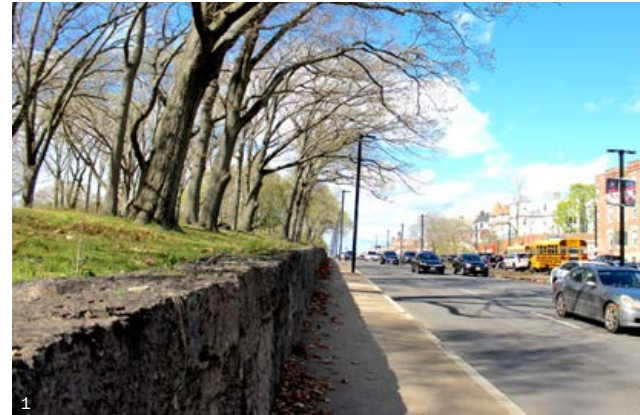
The puddingstone perimeter wall condition.
