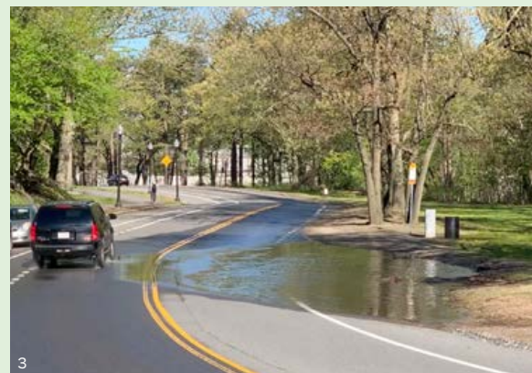
3 Flooding on Circuit Drive after a rain storm.
