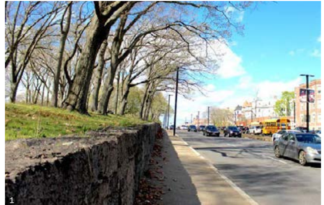
The puddingstone perimeter wall condition.
