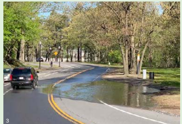
Flooding on Circuit Drive after a rain storm.
