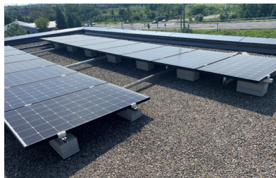
BALLASTED ROOF MOUNTED PV SYSTEM
