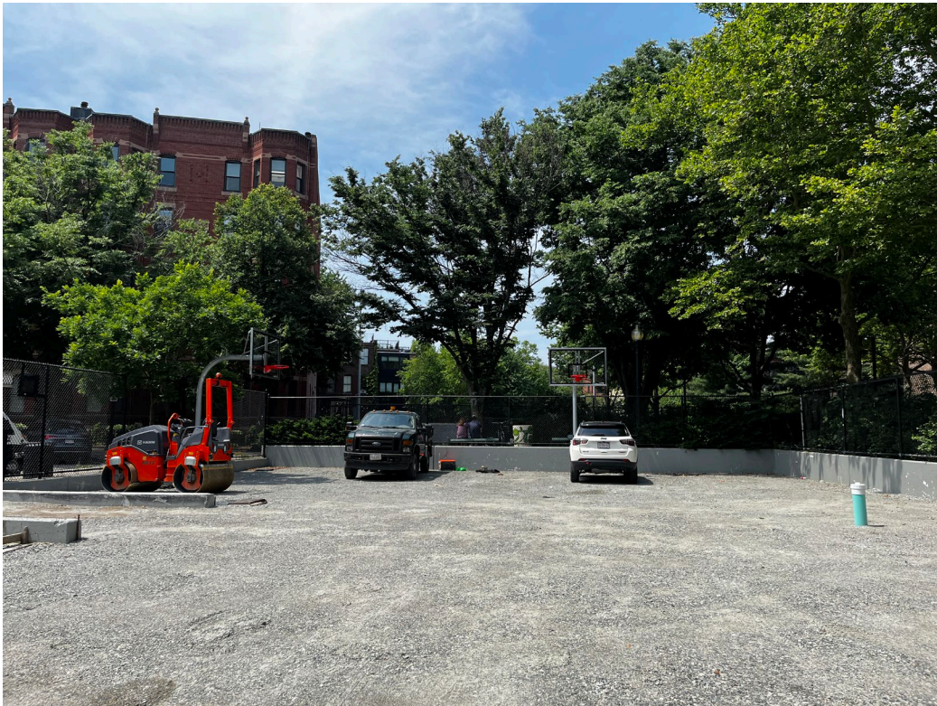
The subsurface drainage system at the basketball court is complete and compaction testing has been completed; paving and surfacing are next!
