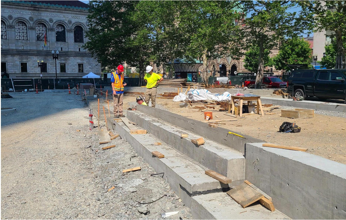
A set of steps that will lead up to the Raised Grove. This is the concrete base - attractive precast concrete steps will be installed on top of this.
