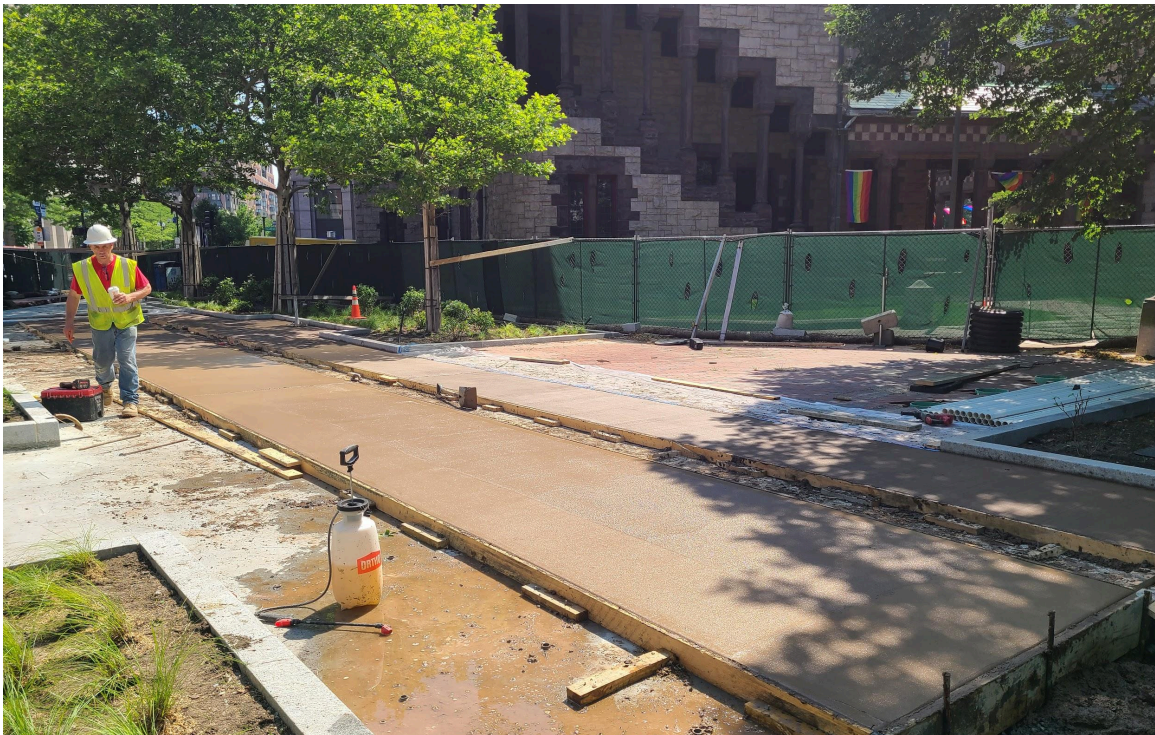
Colored panels of concrete will alternate with bands of unit pavers (installed next!) along the site pathways. Here is the installation of the concrete at the Huntington path, north of Trinity Church.
