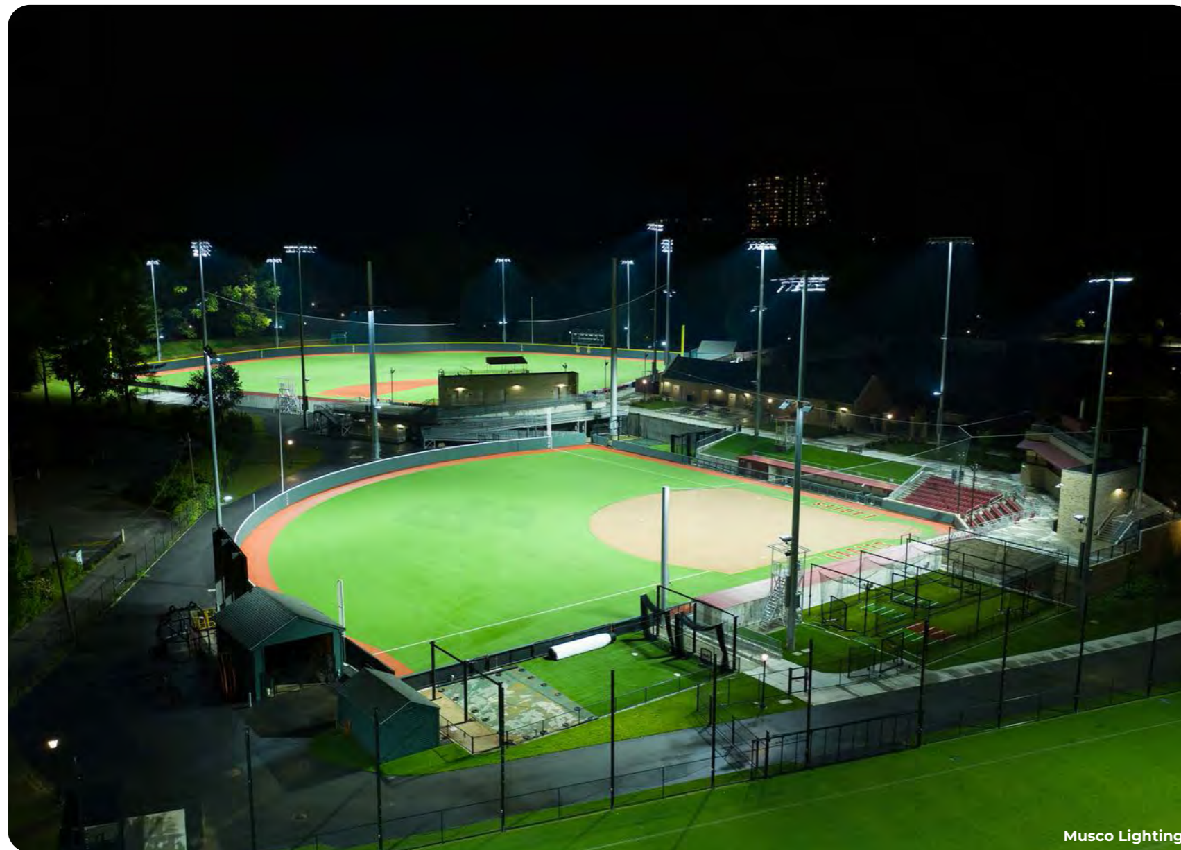
Boston College LED field lights at the Brighton Campus.
