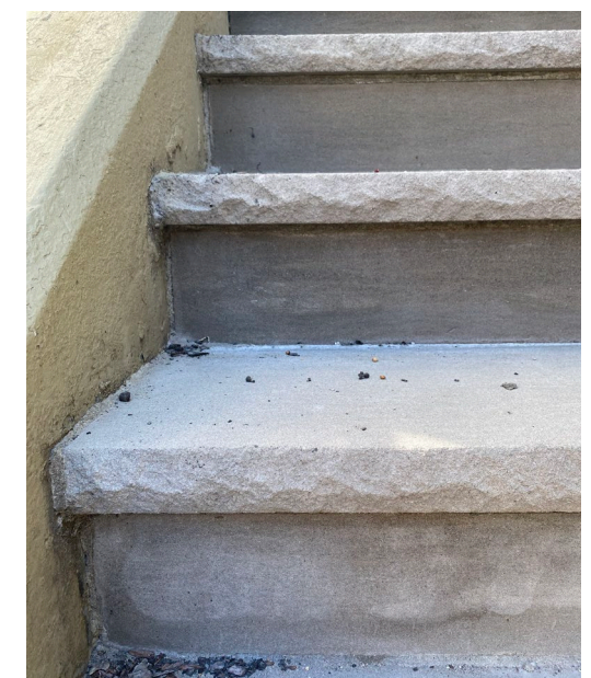
1615 Tremont St – Riser and Tread
