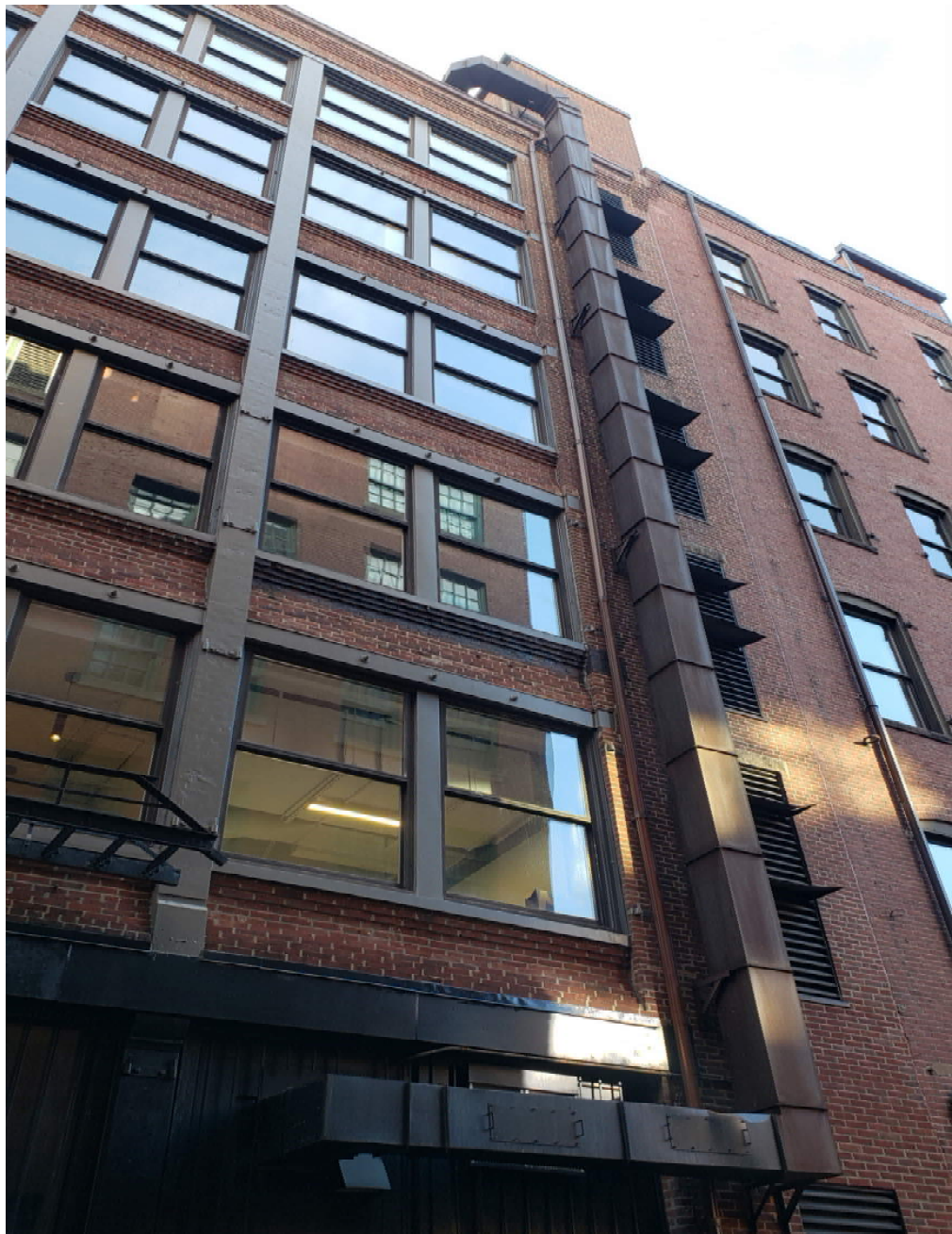
SURFACE MOUNTED DUCTWORK BEHIND "METRO" SPACE
