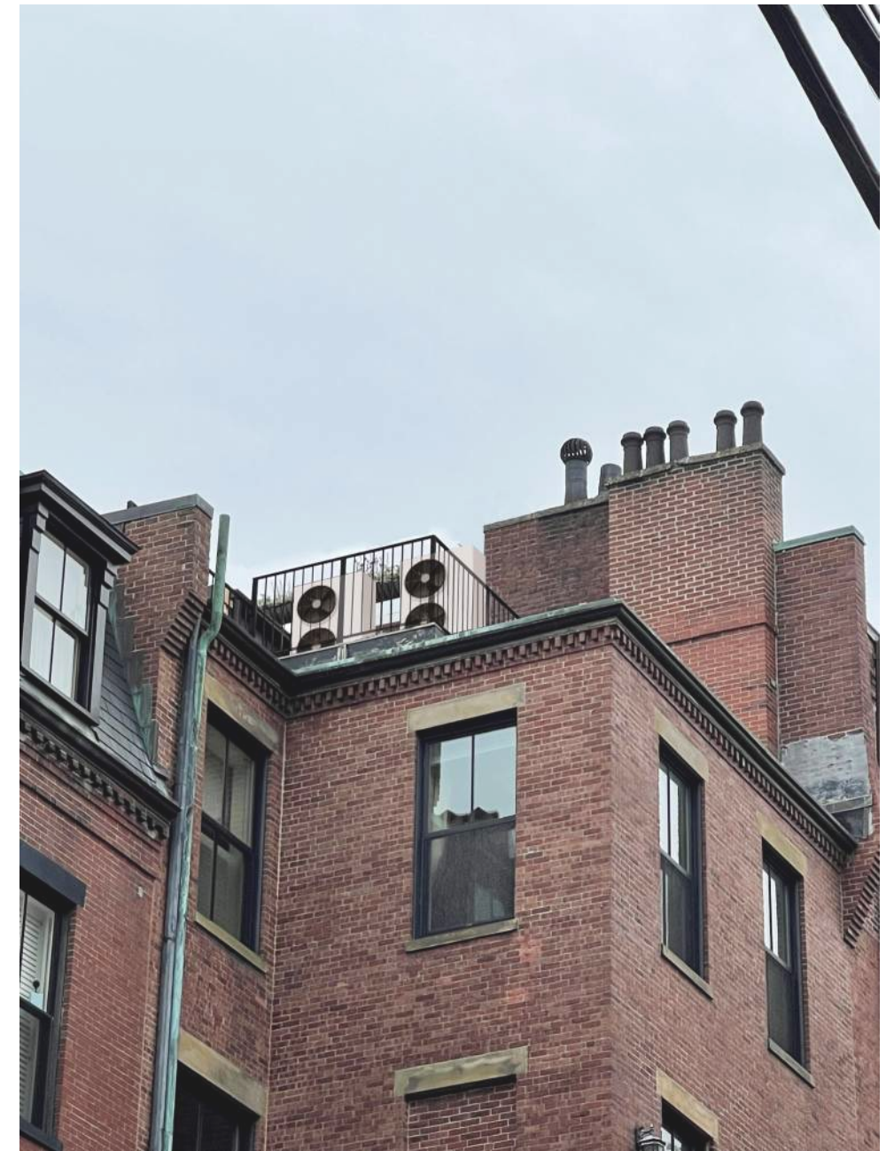
STACKED, NO ENCLOSURE
