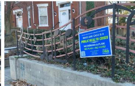
1.6 Outdated style, fading paint at decorative metal fence
