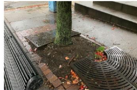
1.3 Tree grate not adjusted for tree growth. Tree is root-bound and heaving paving and grate
