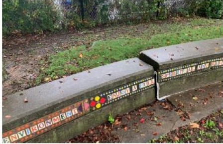
1.3 Damaged mosaic inlays on concrete seat wall
