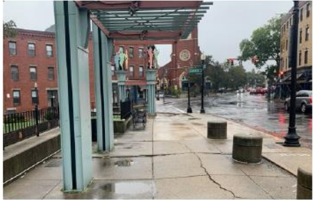
1.2 Bollards and shade structure do not contribute to bus stop and restrict site lines in park. Cracking and heaving of concrete paving. Outdated style.
