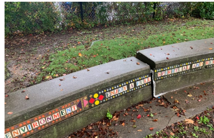
1.3 Damaged mosaic inlays on concrete seat wall
