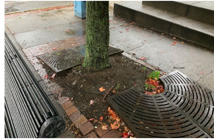
1.3 Tree grate not adjusted for tree growth. Tree is root-bound and heaving paving and grate
