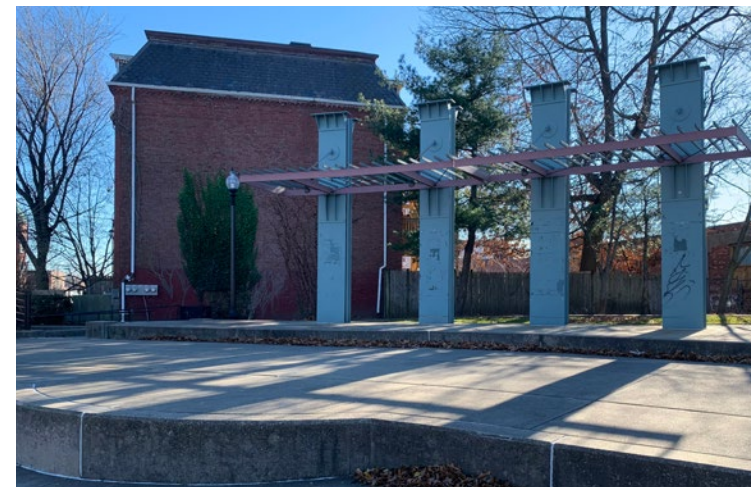
1.5 Fading paint at stage back-drop, outdated style, non-functioning lights
