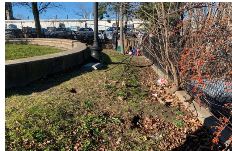
1.5 Overgrown and unmanaged vegetation along back retaining wall and fence
