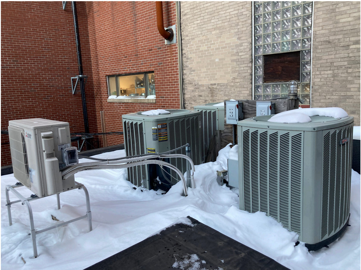
7 - 9 Newbury Street Rear Alley Roof Existing Compressors
