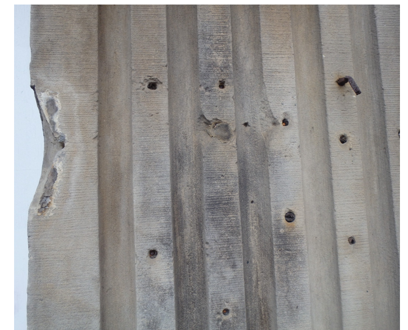
LIMESTONE DAMAGE AT WASHINGTON STREET ENTRANCE
