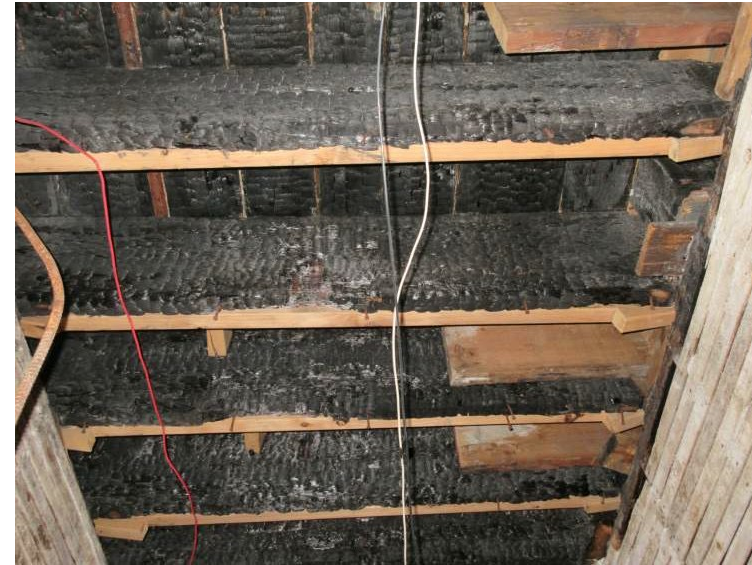
FIRE DAMAGE AT FLOOR FRAMING
