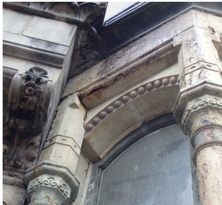
CRACK IN CAST IRON STOREFRONT
