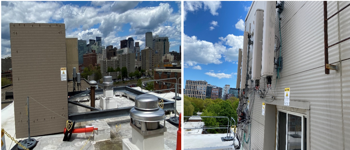
Existing canister and antennas
