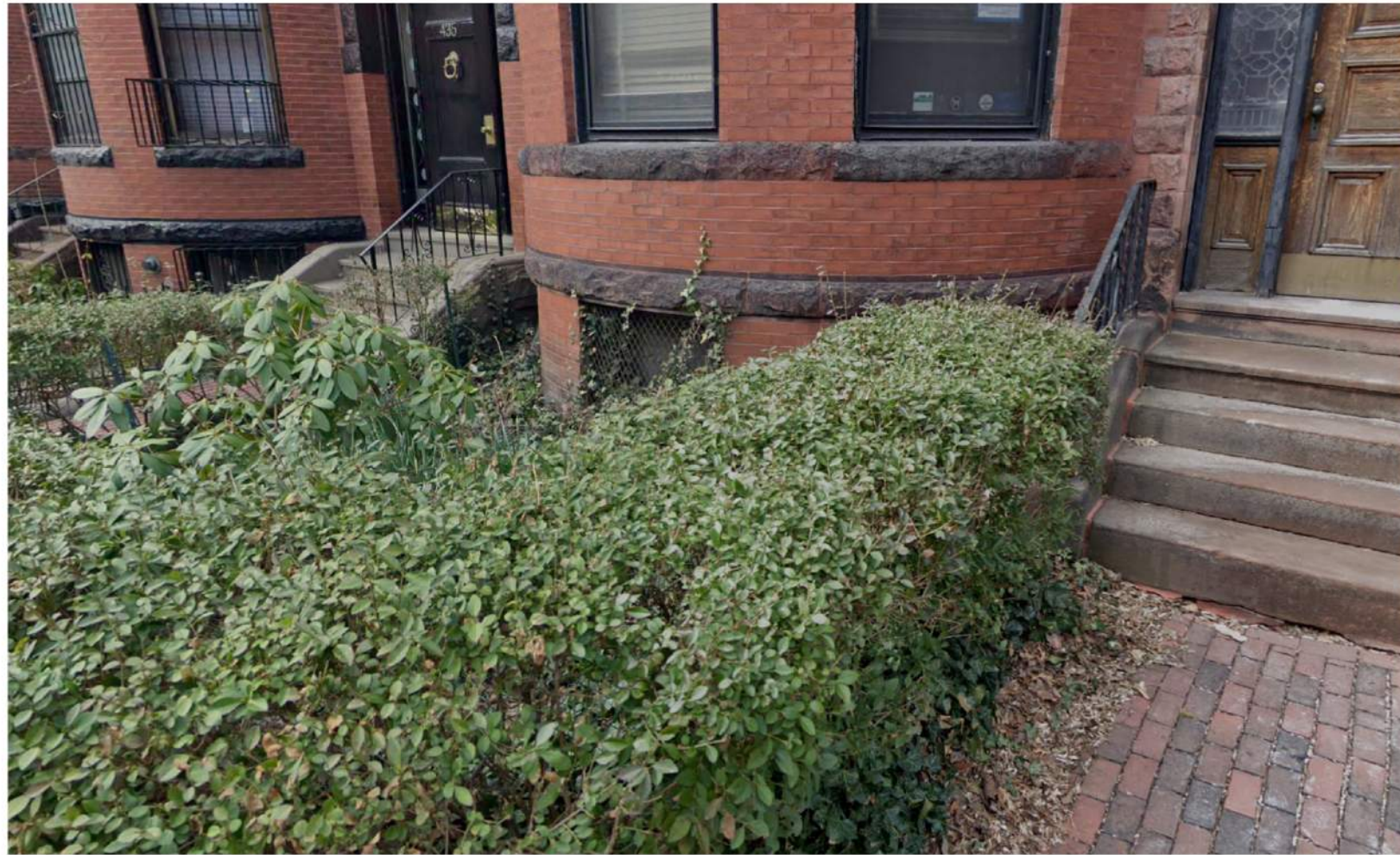
EXISTING WINDOW CONDITION AT 433 MARLBOROUGH ST
