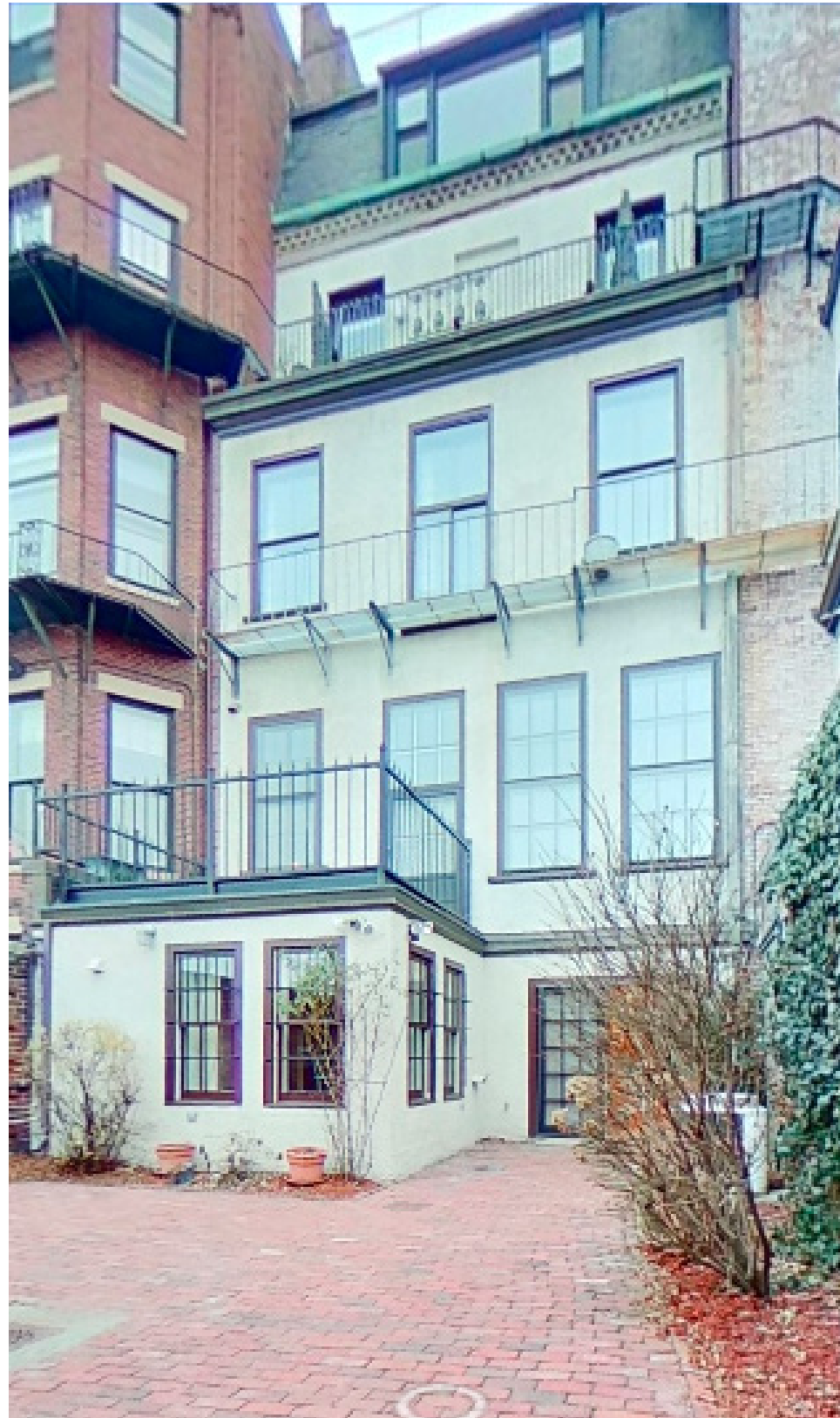
B. NORTH FACADE - PROPOSED WORK TO UNIT 1 (FIRST FLOOR LEVEL AND COURTYARD LEVEL)
