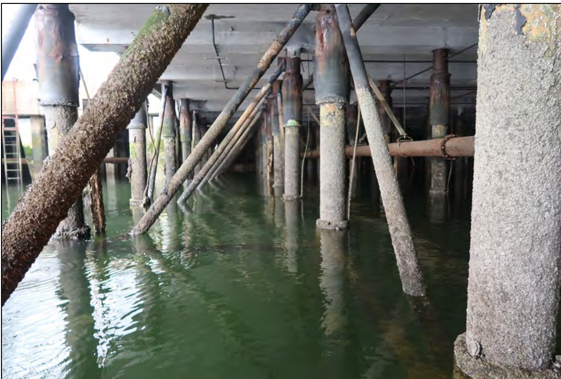
Photo 18 – View of the outer support piles and braces beneath Wharf 3 looking west.
