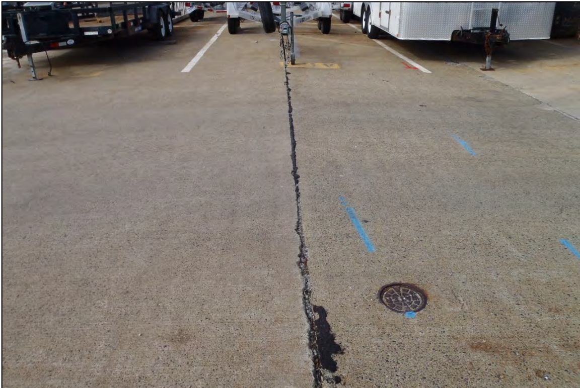
Photo 9 – Spalling of the expansion joint at Wharf 3 looking south.
