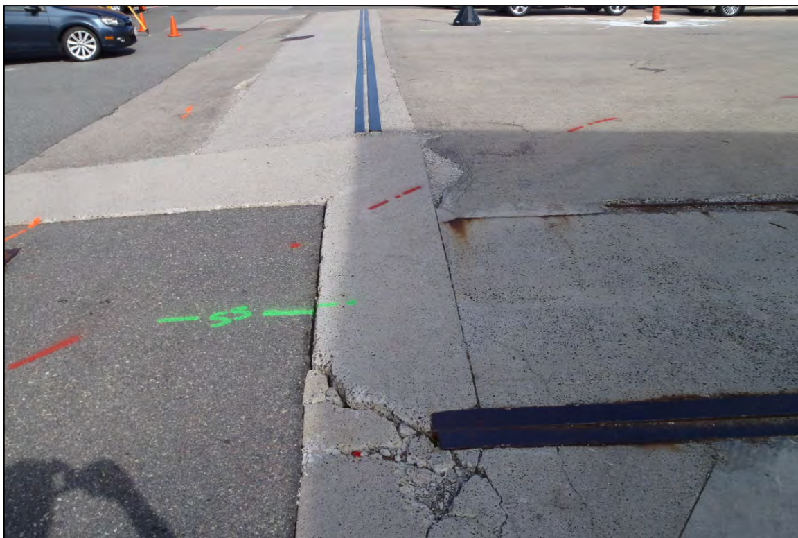
Photo 10 – Spalling around a joint near the western end of the concrete deck of Wharf 3.
