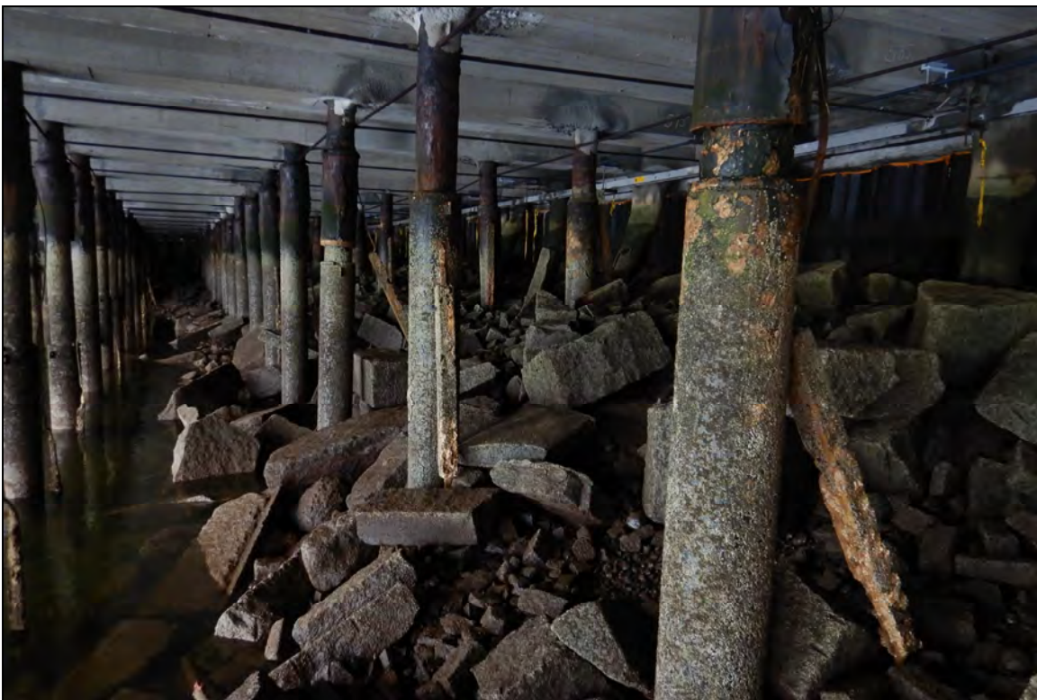
Photo 16 – View of the support piles and riprap slope beneath Wharf 3 looking northwest.
