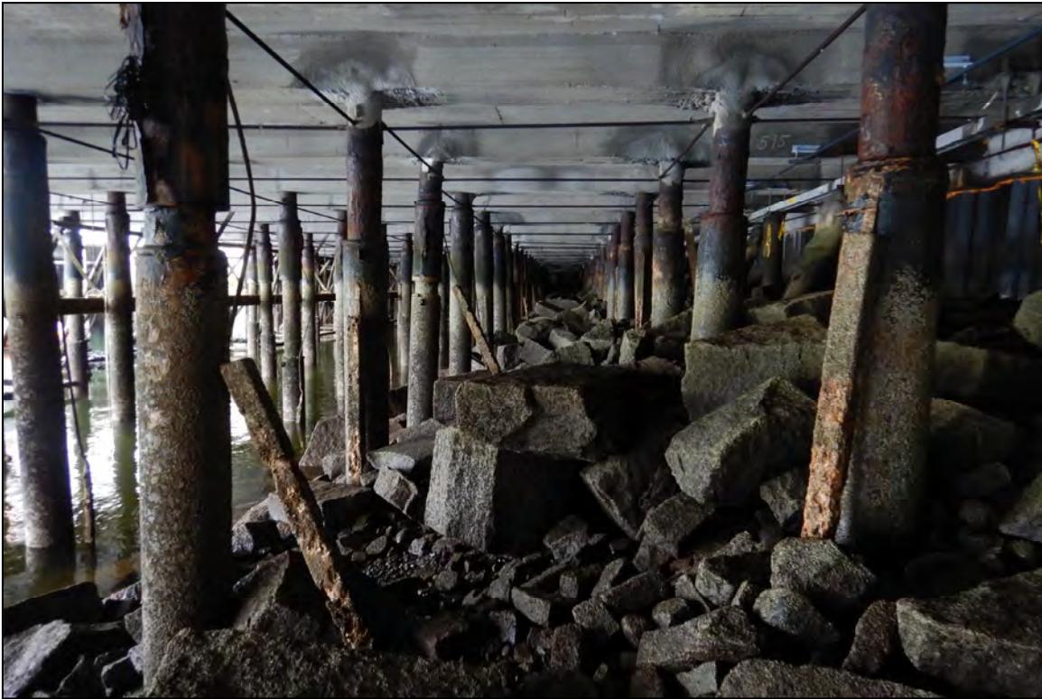
Photo 15 – Overview of the support piles and riprap slope beneath Wharf 3 looking west.
