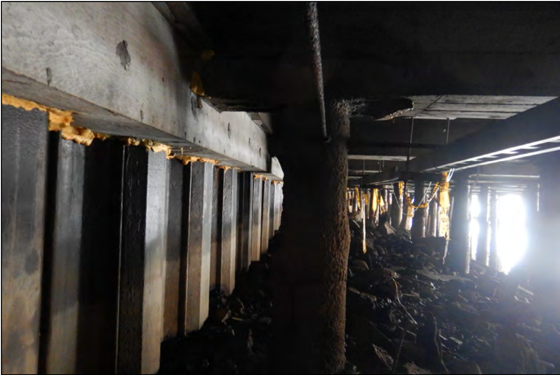
Photo 13 – View of the bulkhead, riprap slope, and piles beneath Wharf 3 looking east.
