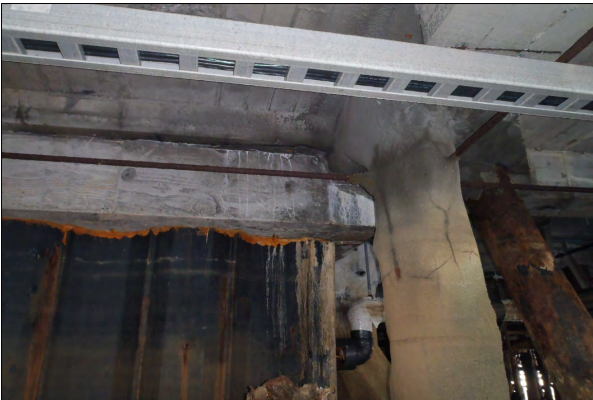
Photo 14 – Corrosion at the corner of the bulkhead beneath Wharf 3.
