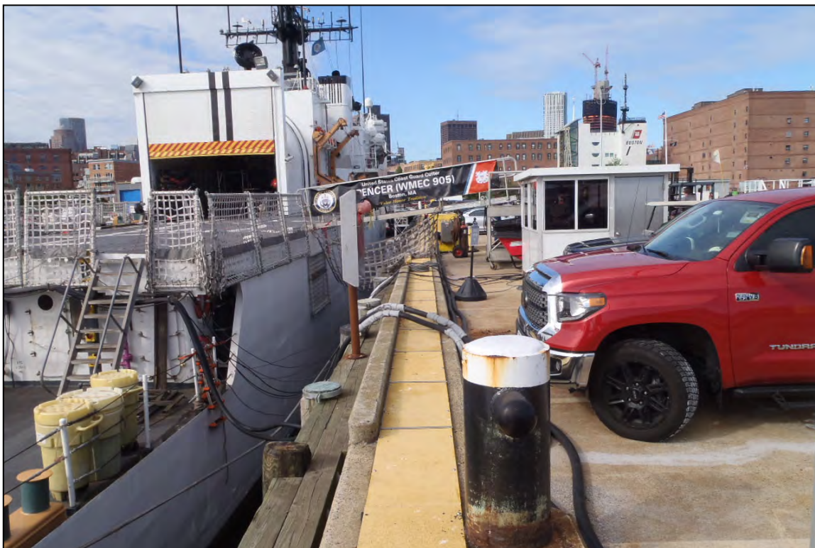
Photo 5 – View of the curb and fender system along the south side of Pier 2 looking west toward Wharf 3.
