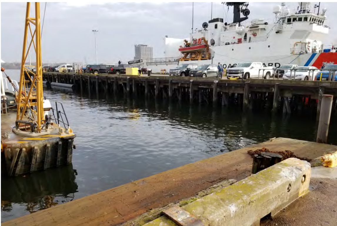
Photo 3 – View of the fender system along the north side of Pier 2 looking south.
