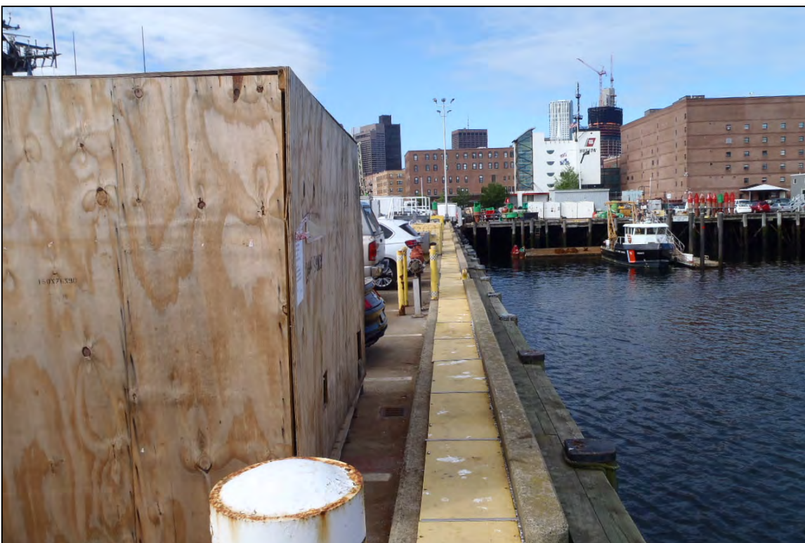
Photo 4 – View of the fender system along the north side of Pier 2 looking west.
