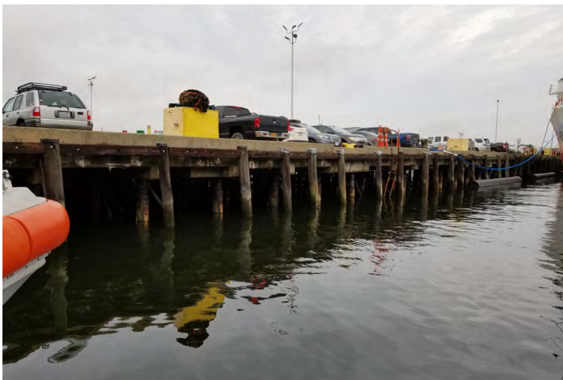
Photo 6 – View of the fender system along the south side of Wharf 3 looking northeast.
