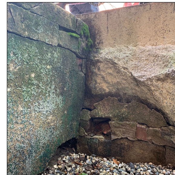
3 WINDOW WELL EXISTING CONDITIONS IN NEED OF REPAIR / PARGING
