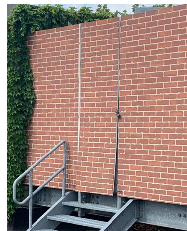
Existing faux brick to be replaced
