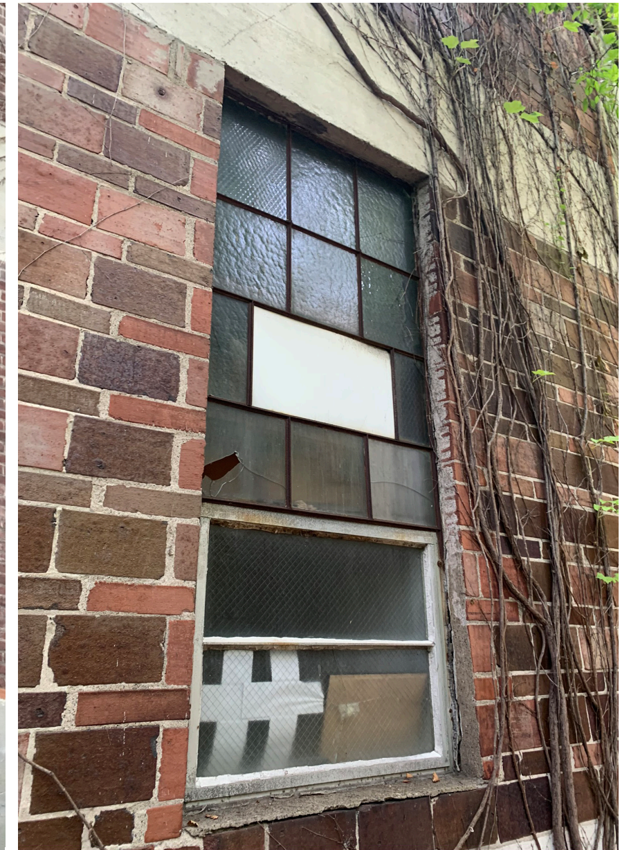
Existing damaged window on south facade
