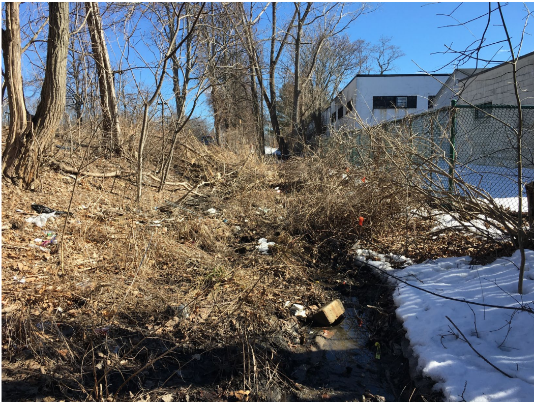
View to East up the Drainage Showing Fence, Various Debris, and Vegetation Overgrowth
