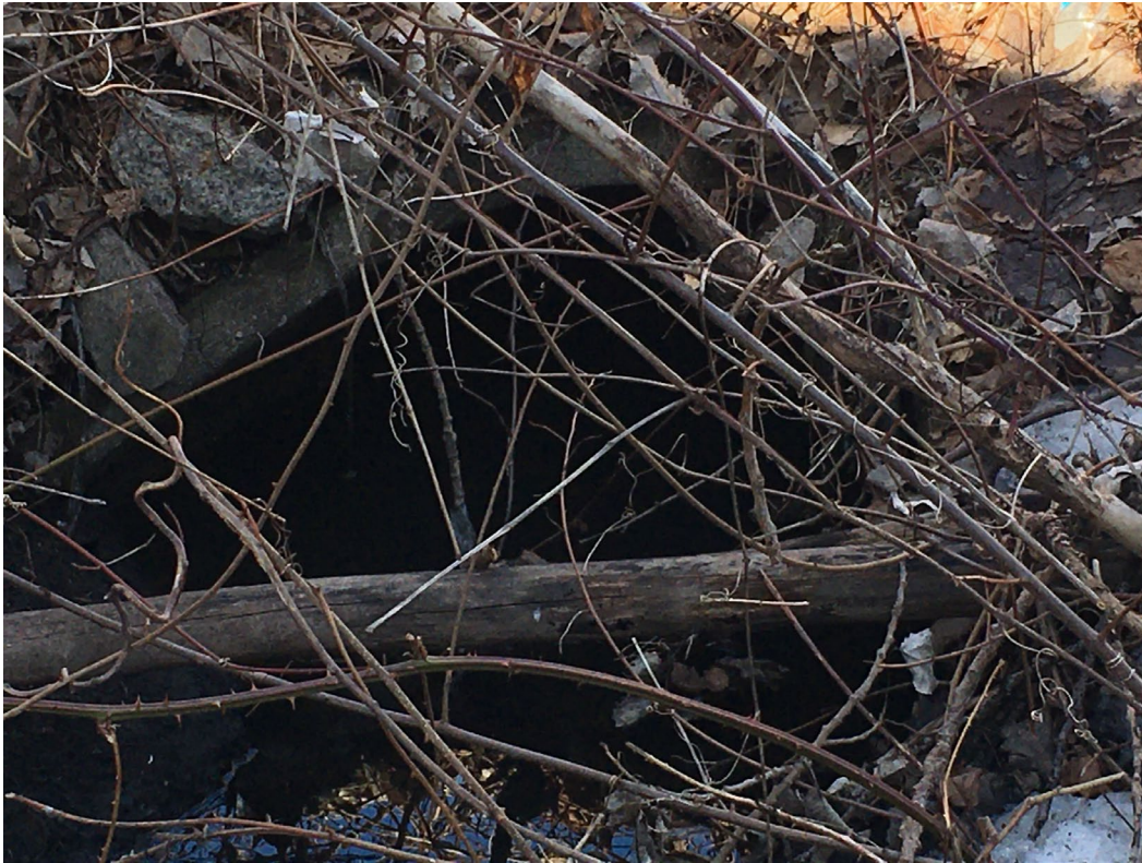
View to North of RCP Outfall at Head of Drainage from Home Depot
