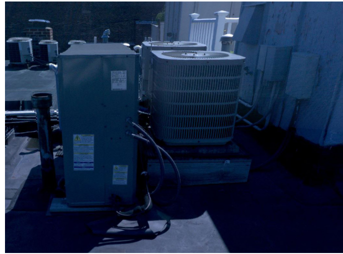
existing roof top units
