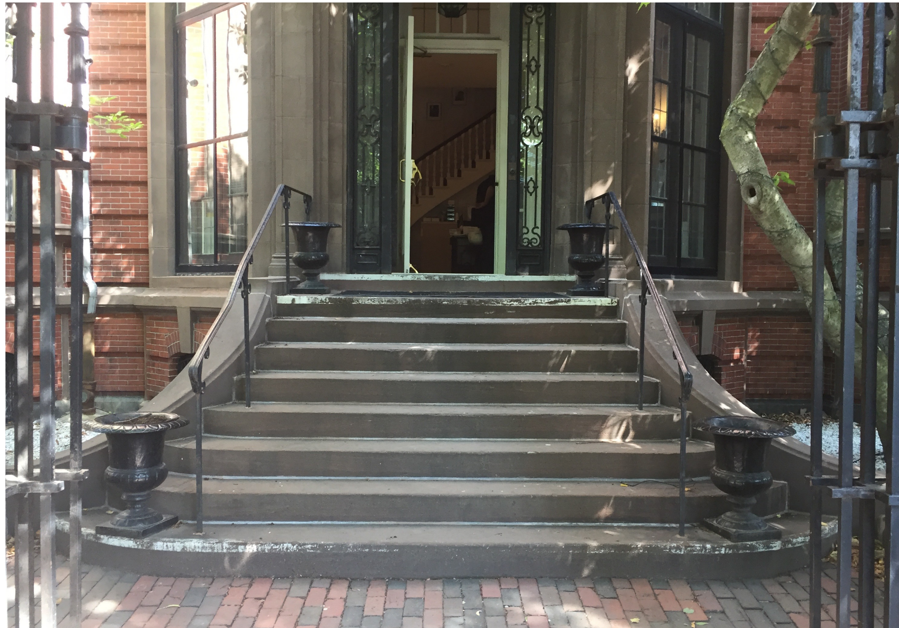
VIEW OF EXISTING HAND/GUARDRAIL TO BE REPAIRED/REPLACED
