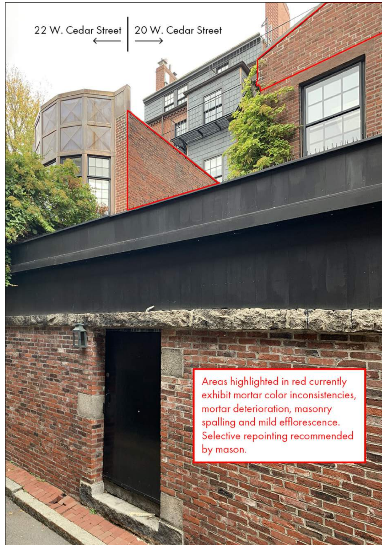
2 EXISTING VIEW 4 - REAR FACADE REQUIRING SELECTIVE REPOINTING (VISIBLE FROM CEDAR LANE WAY)
