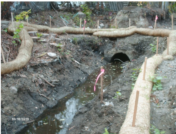
South drain ditch and outfall pipe.
