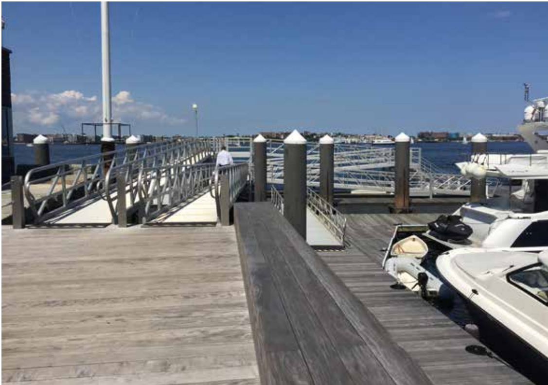
Harborwalk, gangway, wave attenuator, and western float in the northwestern portion of the Project Site
