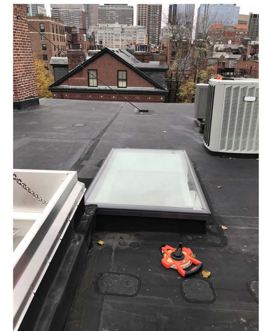
EXISTING SKYLIGHT AND A/C CONDENSERS
