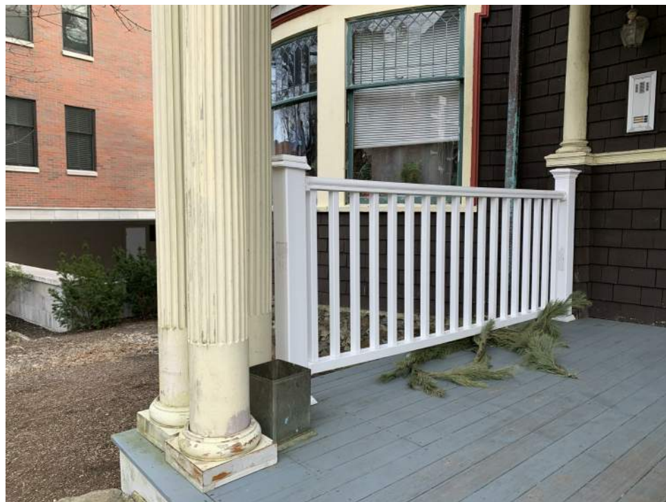
EXISTING NON-HISTORIC PVC GUARD RAILING AT 38 ENGLEWOOD
