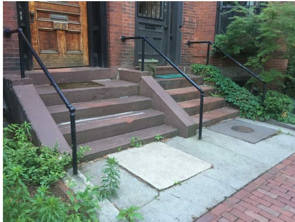
25-23 CUMBERLAND - PIPE RAIL AT STOOP; NO GARDEN RAILS
