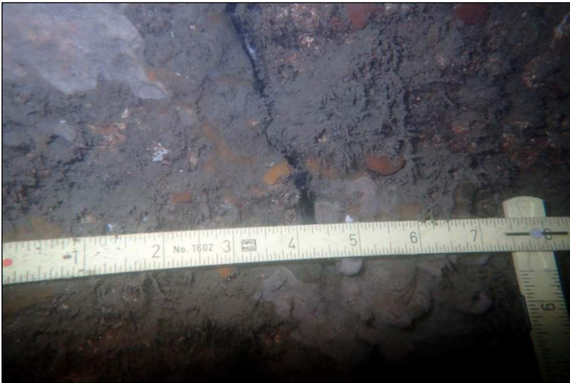
Photograph 4: Typical Cracked Granite Block Underwater.
