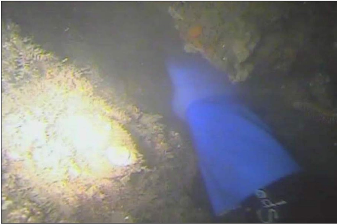
Photograph 3: Significant Void at Mudline Due to Displacement of Blocks (Sta. 10+40).
