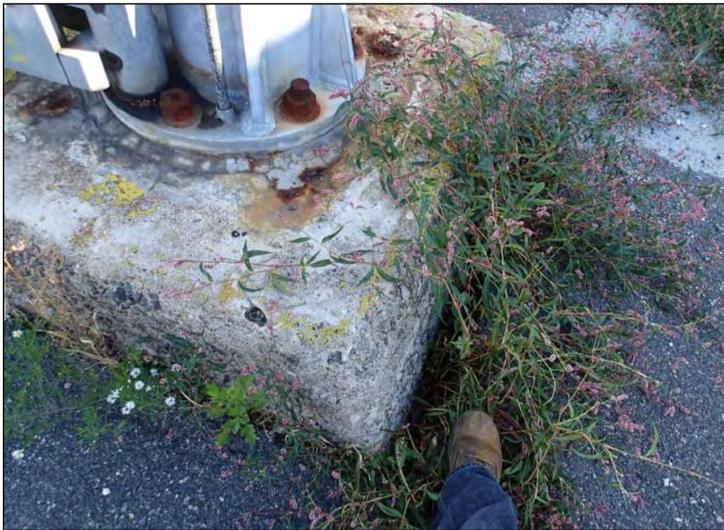
Photograph 6: Mooring Hook Foundation Displacement in the Offshore Direction
