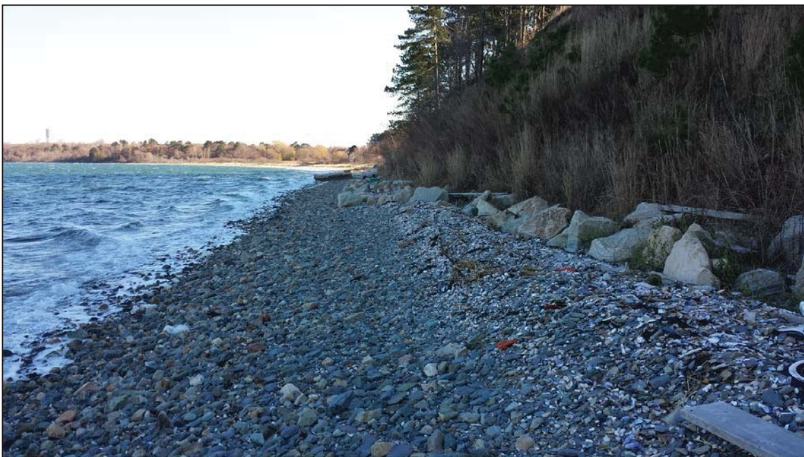
Photo 2: View northeast of the coastal bank and coastal beach on the northern side of the Long Island Bridge approach on Long Island in Boston, MA.
