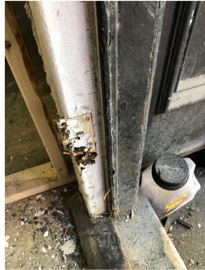
EXISTING JAMB: HINGES PULLED OUT FROM JAMB DUE TO ROT AND WATER DAMAGE
