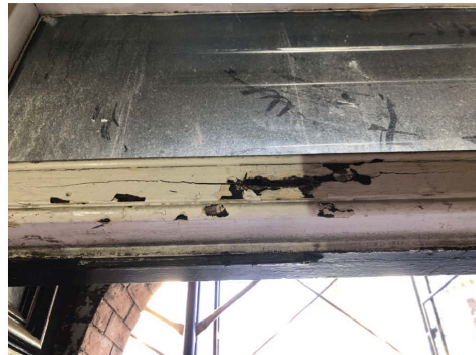
EXISTING HEAD JAMB: JAMB IS SPLIT DUE TO WEIGHT/STRESS OF HEAVY DOORS, ROT AND FAILING DOOR UNIT.
