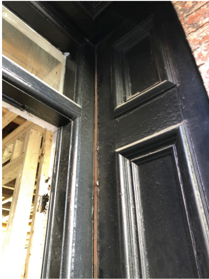
EXISTING JAMB/PANEL: PANEL AND JAMB HAVE SEPARATED WITH REPEATED USE DURING CONSTRUCTION
