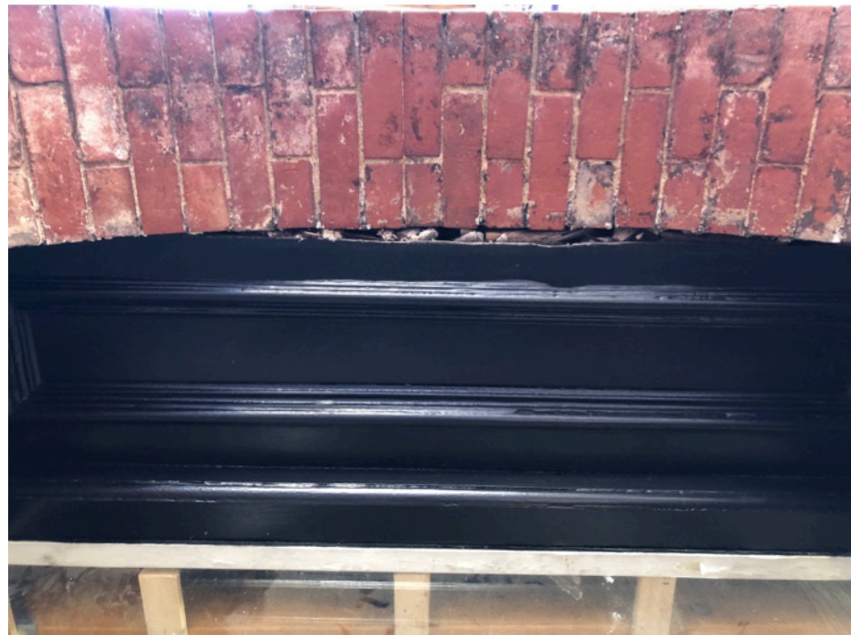
EXISTING CEILING PANEL: GAP AT CEILING PANEL TO BRICK WALL, NEEDS TO BE REBUILT TO PREVENT WATER DAMAGE
