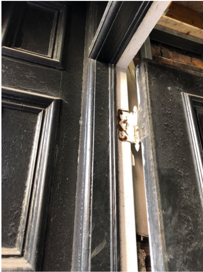
EXISTING JAMB: WATER DAMAGE AROUND MOULDINGS
