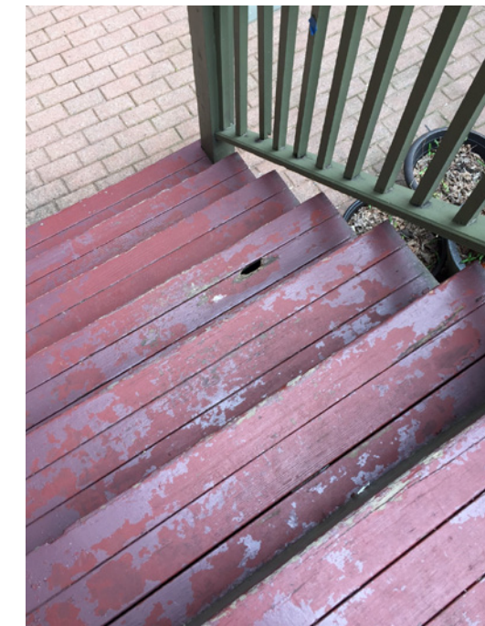
Existing stair damage
