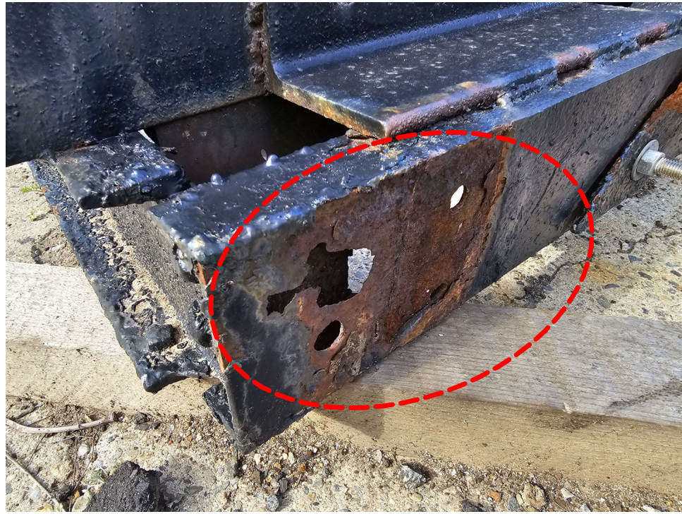
CONSIDERABLE SECTION LOSS ON STEEL MEMBER
