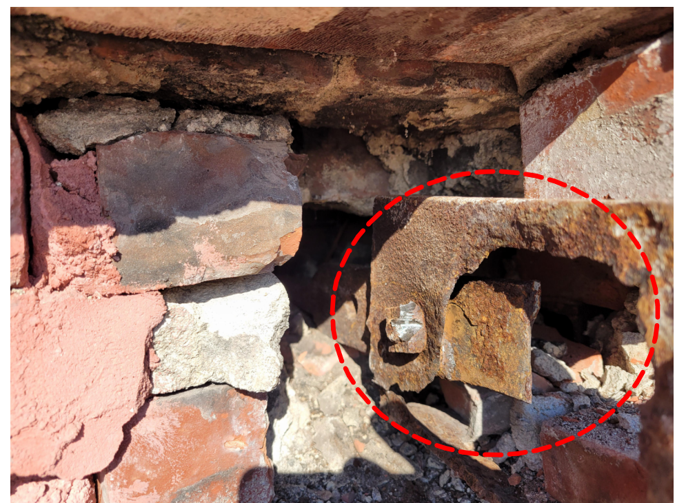
STEEL CHANNEL DETERIORATION - CONSIDERABLE SECTION LOSS DUE TO RUST SCALING
