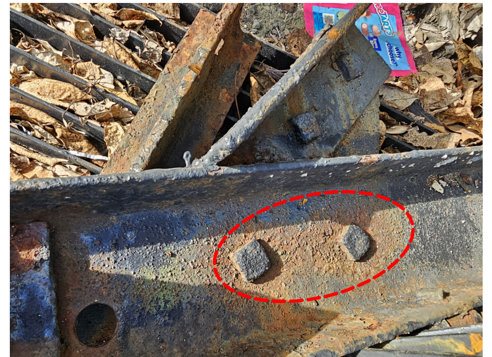
SQUARE BOLT FROM THE 70'S NO LONGER USED. CURRENTLY, THERE IS NO TOOL TO PERFORM PULL TEST ON THESE BOLTS
