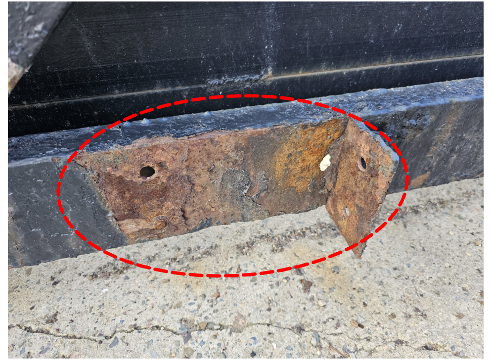
CONSIDERABLE SECTION LOSS ON STEEL MEMBER
