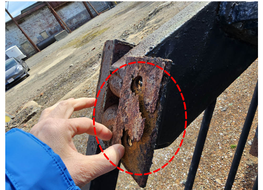
CONSIDERABLE SECTION LOSS DUE TO RUST SCALING
