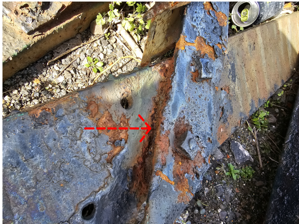
SIGNIFICANT AMOUNT OF RUST SCALING IS MOVING THE STEEL MEMBER OUT OF PLACE
