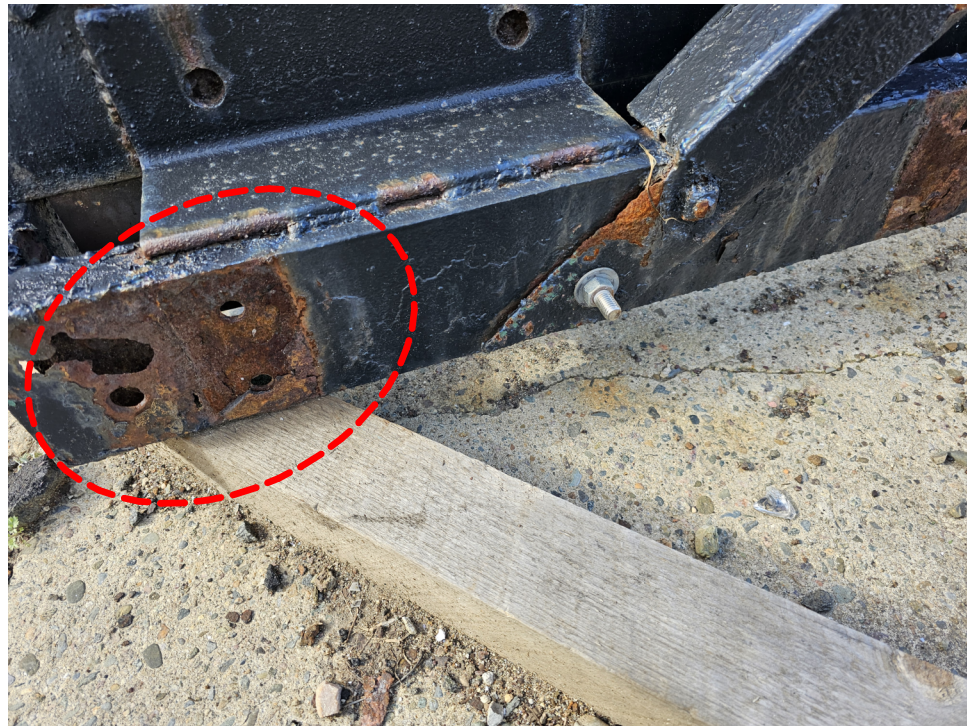
CONSIDERABLE SECTION LOSS ON STEEL MEMBER
