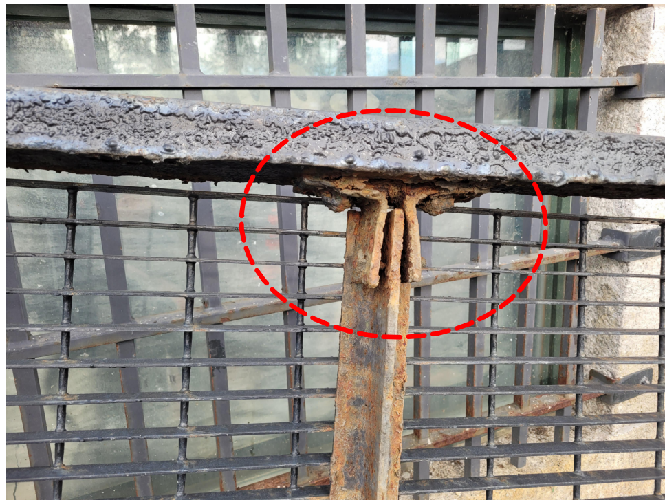
RUST SCALING AT STEEL ANGLES - ANGLES MOVING OUT OF PLACE
