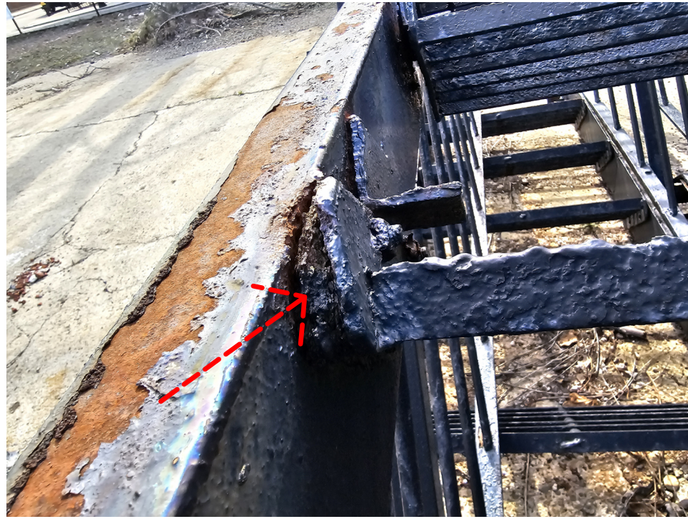
SIGNIFICANT RUST SCALING MOVING STEEL COMPONENTS OUT OF PLACE
