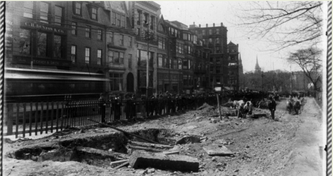
This photo from April 1895 shows the beginning of excavations for the subway in front of Central Burying Ground. The discontinued underground brick tombs are seen in the excavated areas. A crowd of people is gathered outside the fence watching the work.
