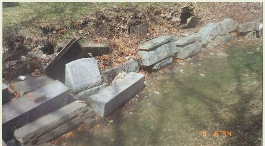
By 1994 the granite blocks in the large tomb structure were pushed outwards and collapsed, leaving tombs open to the public.
