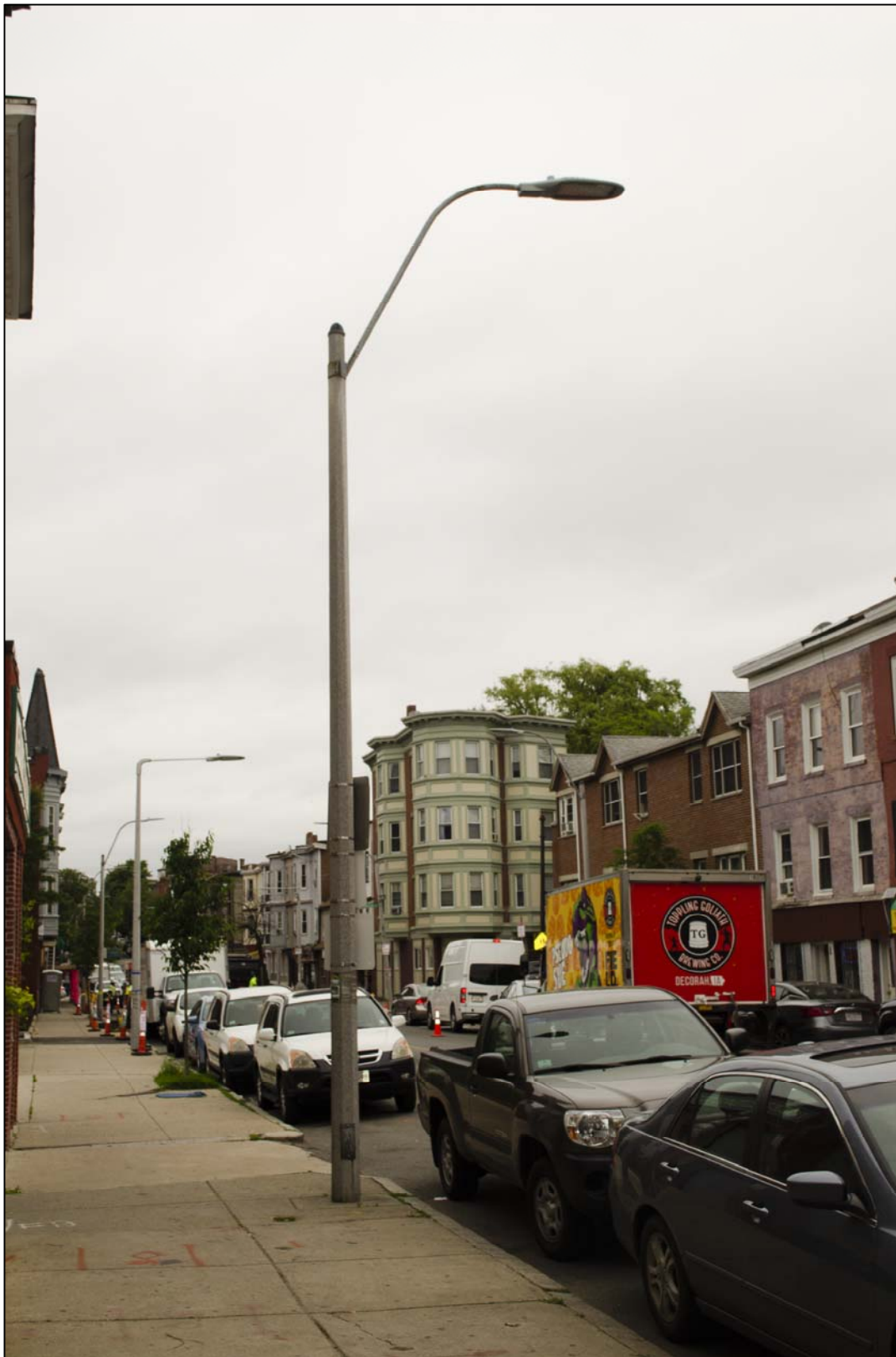
STANDARD CONCRETE LIGHT POLE - COBRA LUMINARY FIXTURE EXISTING CONDITIONS PHOTOGRAPH - EXHIBIT X-1
