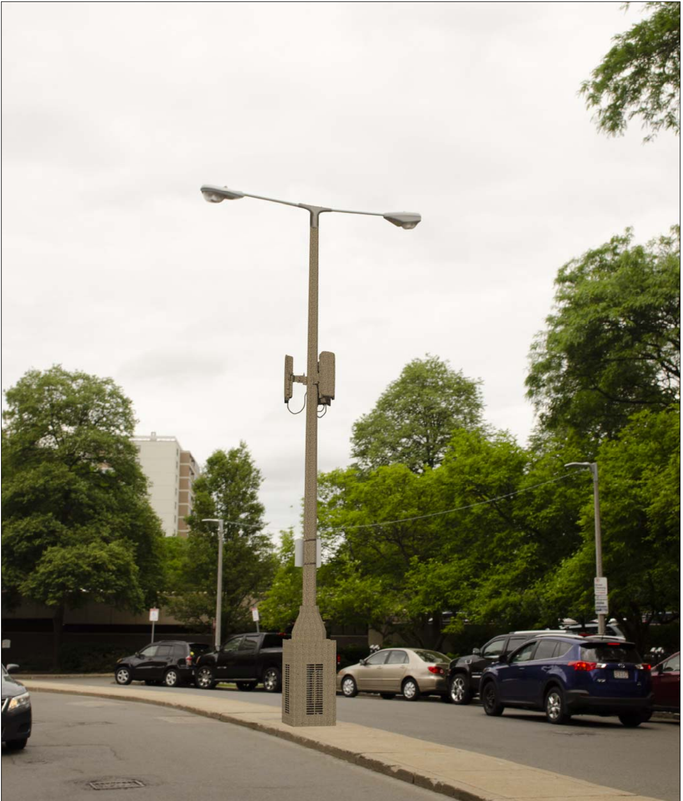
STANDARD CONCRETE LIGHT POLE - DOUBLE STRAIGHT LUMINARY FIXTURE PROPOSED PHOTOSIMULATION - EXHIBIT X-1D
