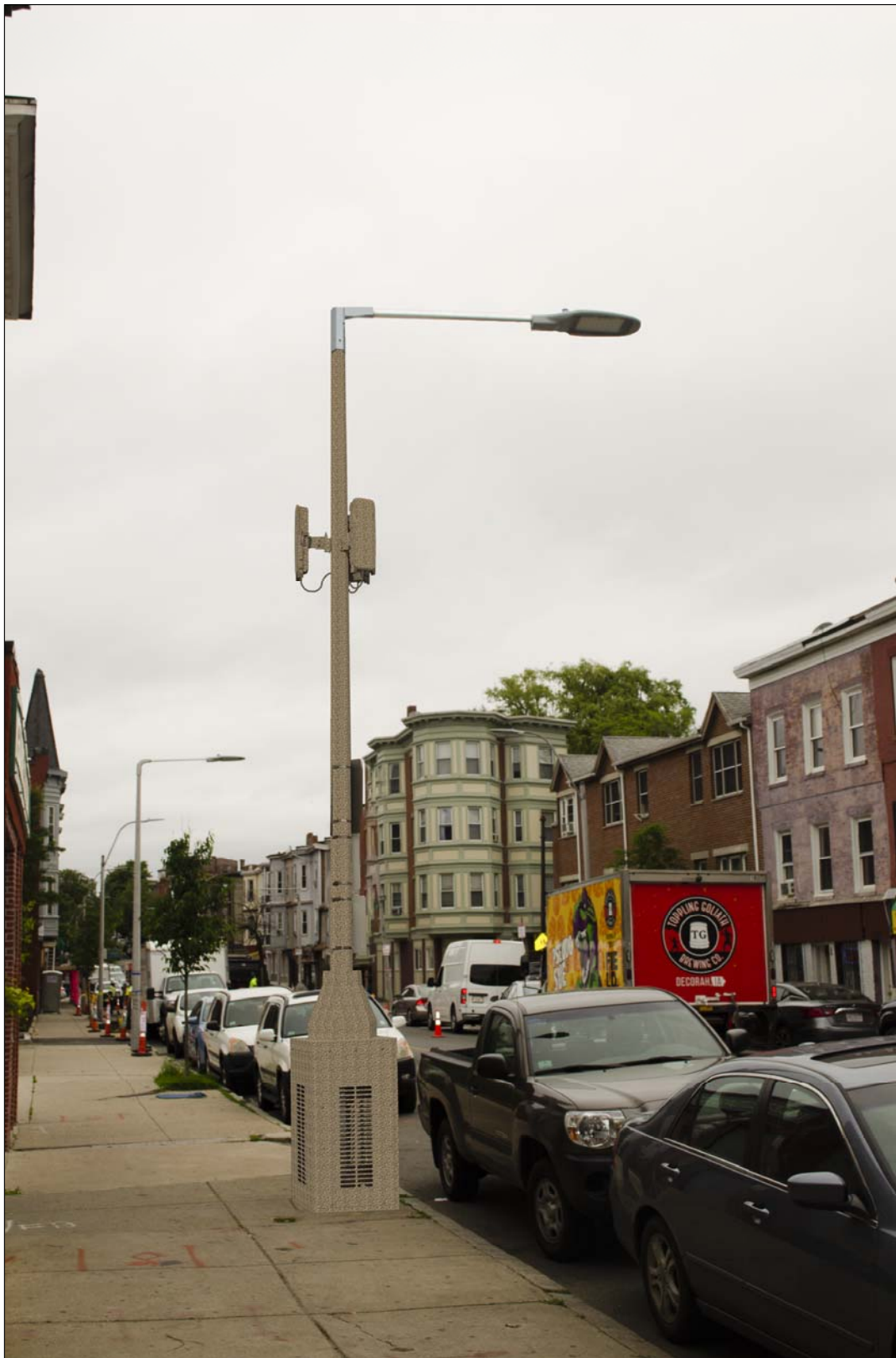
STANDARD CONCRETE LIGHT POLE - EXISTING COBRA LUMINARY FIXTURE PROPOSED STRAIGHT LUMINARY FIXTURE PHOTOSIMULATION - EXHIBIT X-1D
